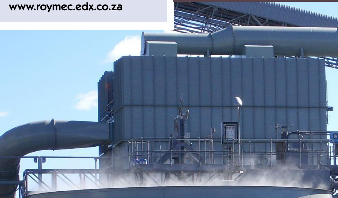
Thickener plant at Rustenburg, South Africa
